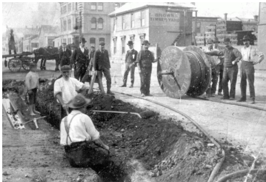
1903 installation of one of the first domestic electricity networks in Christchurch. oooooooooooo
